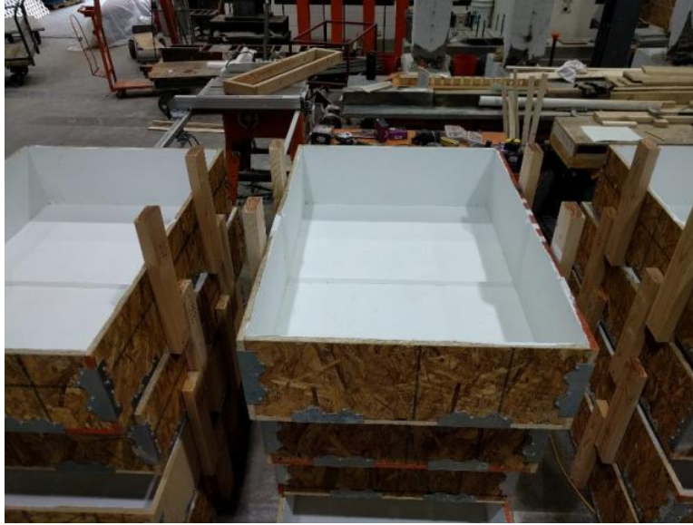
Figure 27 - Assembled and painted formwork without upper brace. Seventeen forms were built in total.
