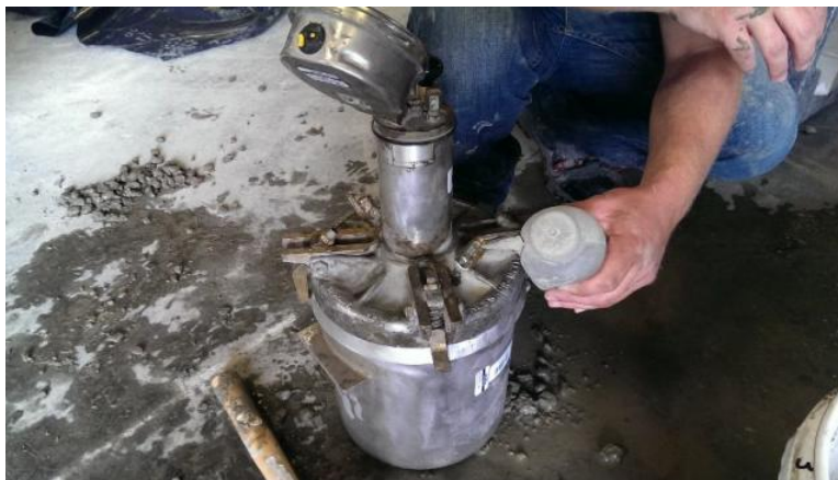
Figure 86 - A small quantity of water and isopropyl alcohol is added just until it begins to run out the weep hole.
