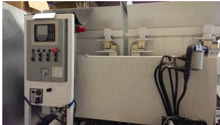
Figure 29 - Close view of mobile batch plant at Fall Line. Note load cells for weighing hopper contents.
